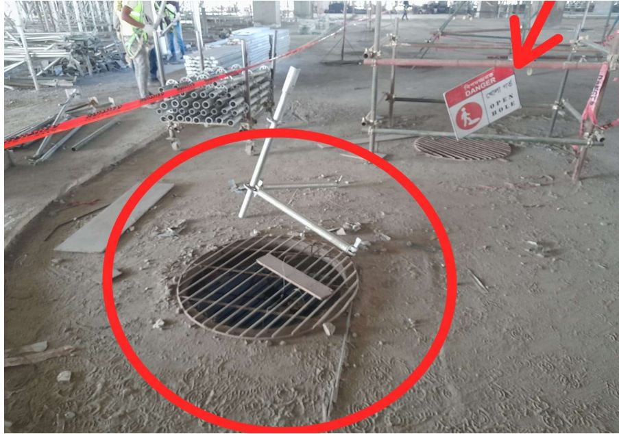
Figure 3.25: No safety barrier provided at floor opening
