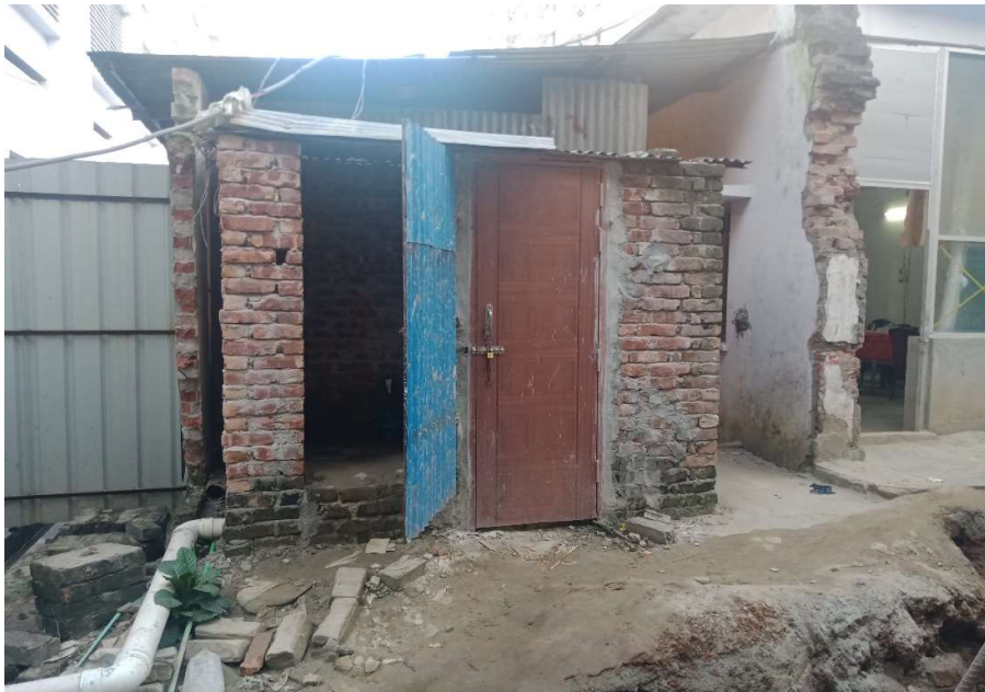
Figure 3.24: Unhygienic toilet at construction site
