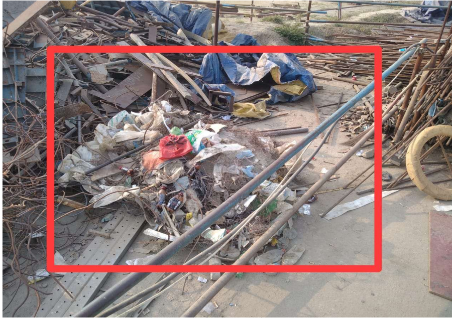
Figure 3.27: Poor housekeeping at workplace
