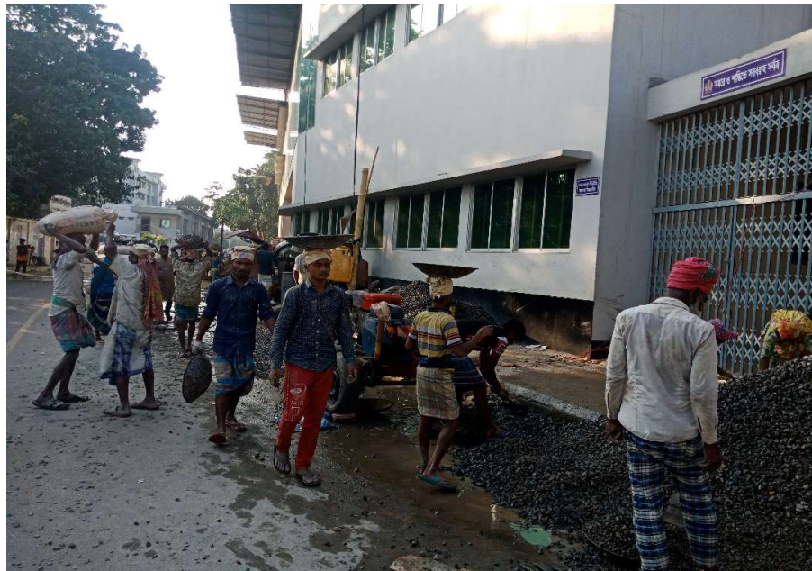
Figure 3.10: Worker working without PPE
