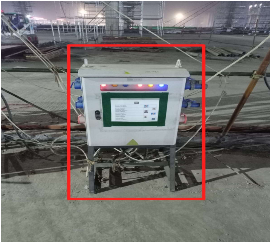
Figure 3.26: No fire extinguisher provided beside electrical box
