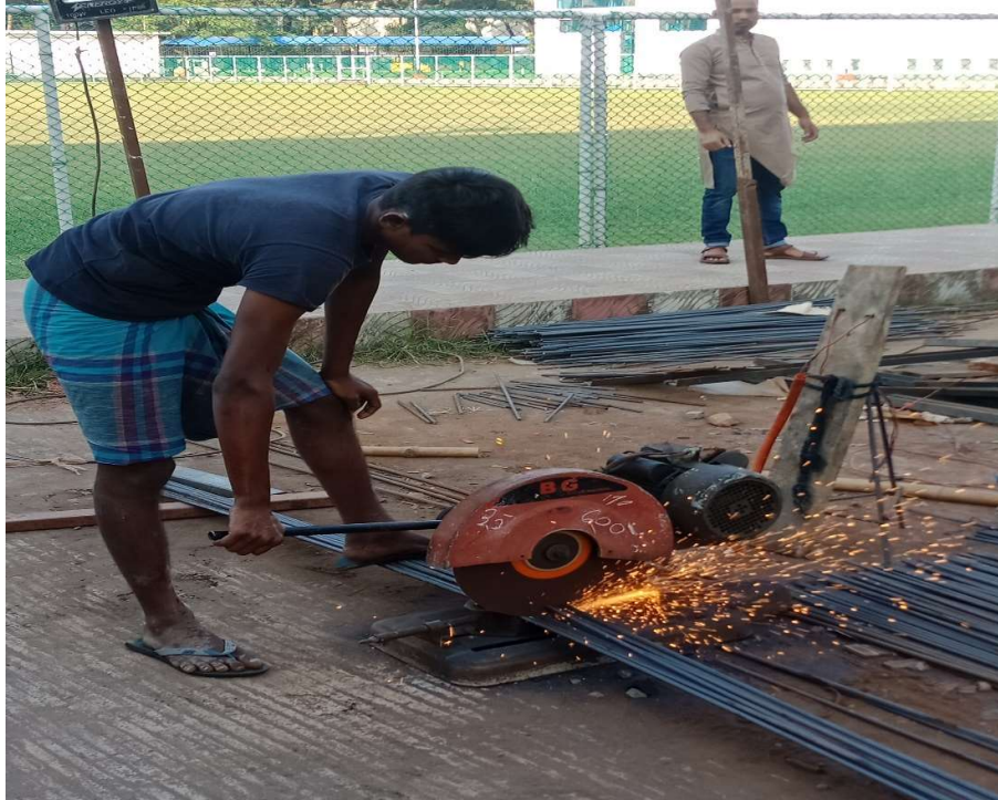
Figure 3.11: Worker Working without hand gloves and eye protection
