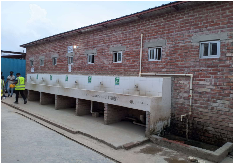
Figure 3.20: Pure water supply and toilet for workers
