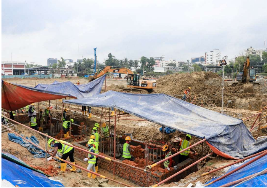
Figure 3.9: Hard safety barrier provided at work place
