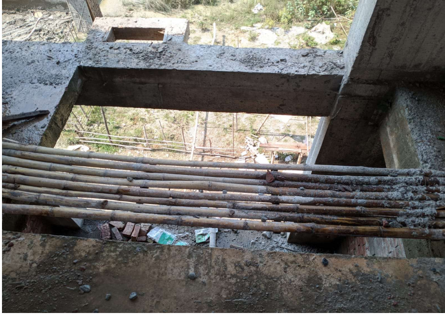
Figure 3.23: No safety barrier provided at floor opening
