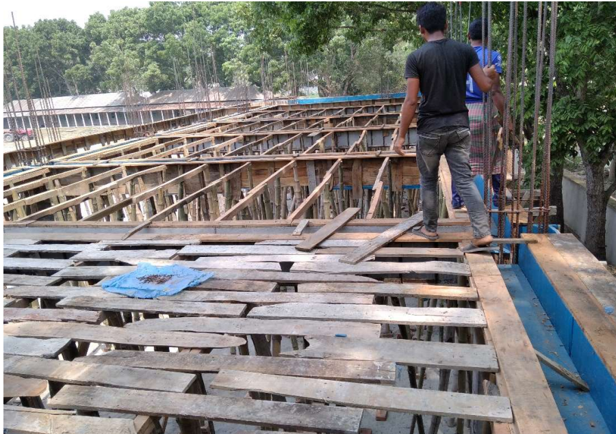
Figure 3.16: Worker working without fall protection
