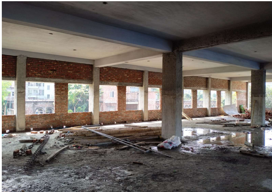
Figure 3.18: Poor housekeeping at construction site
