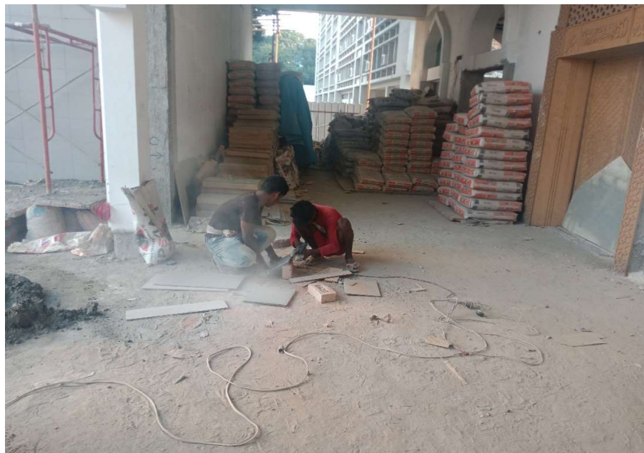
Figure 3.12: Worker working without hand gloves and eye protection
