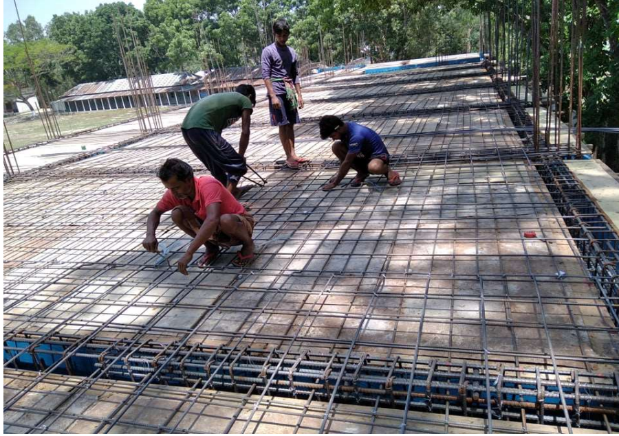
Figure 3.15: Worker working without PPE
