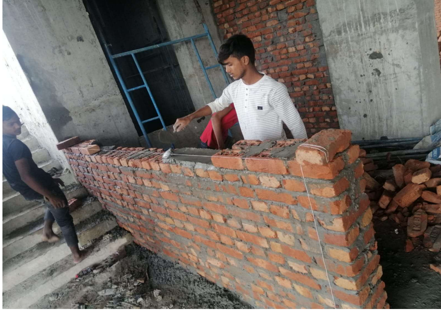
Figure 3.13: Worker working without safety
