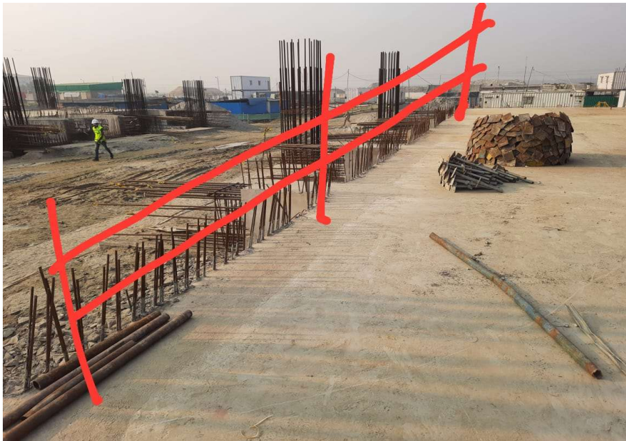
Figure 3.28: No hard barrier provided at danger area
