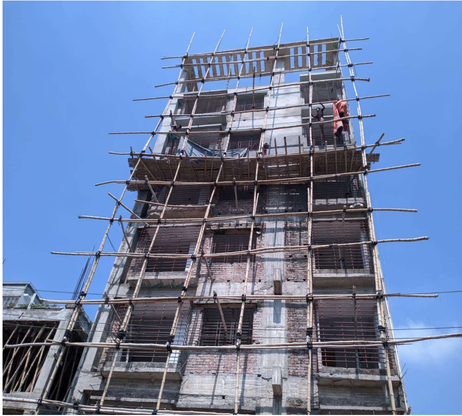
Figure 3.19: No safety barrier, safety shade and staging at site
