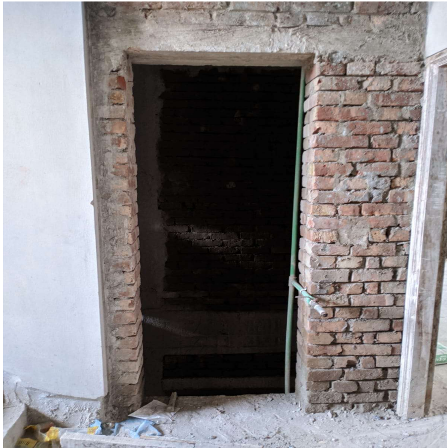
Figure 3.21: No safety barrier at lift opening
