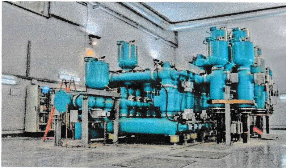
Fig 1.7: Gas Insulated Substation
