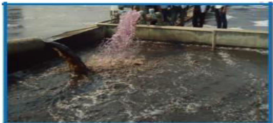
Fig: Sludge from recycle tank
