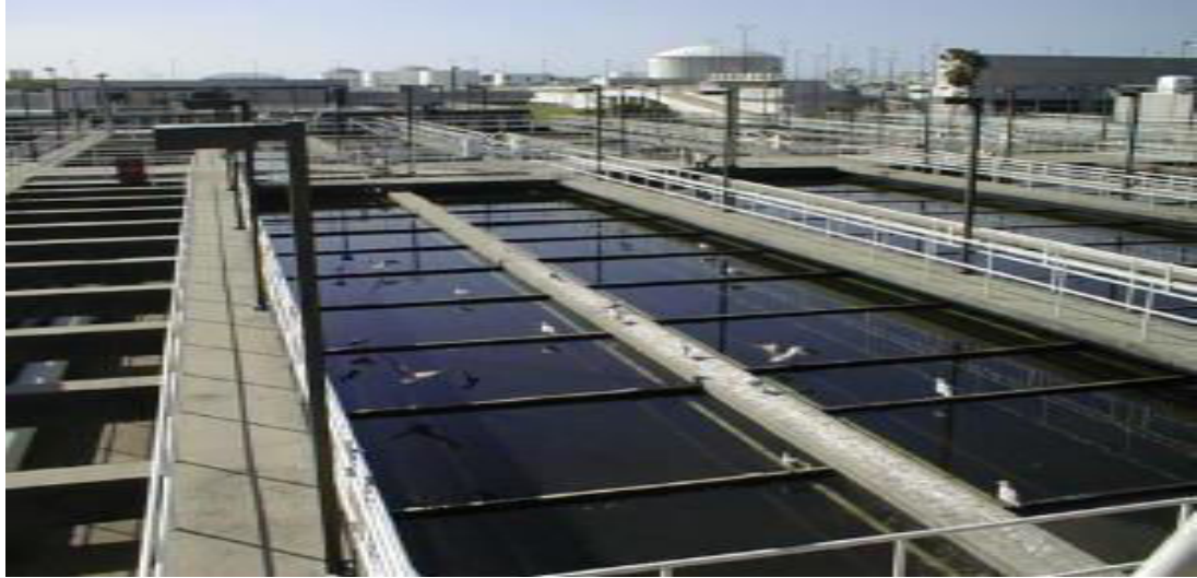
Fig: Discharge to sedimentation tank
