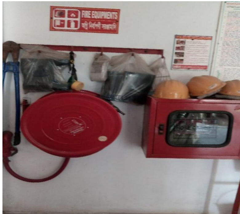
Picture 3.6.3.1. Fire equipment
