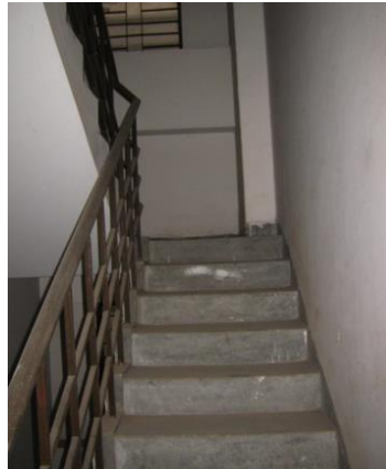
Figure 2: Emergency stair for fire (Length is to small)
