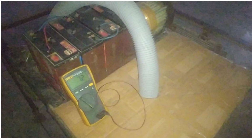
Figure 16: Temperature reading record from backup Air conditioning system
