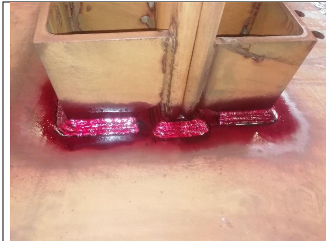
Penetrant of stub Leg
