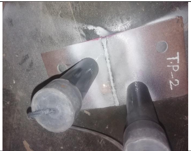
MPI of Welding Plate
