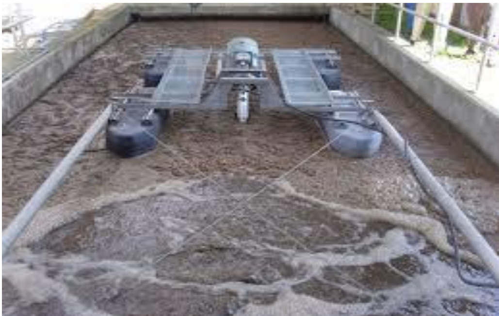
Figure: Equalization tank View
