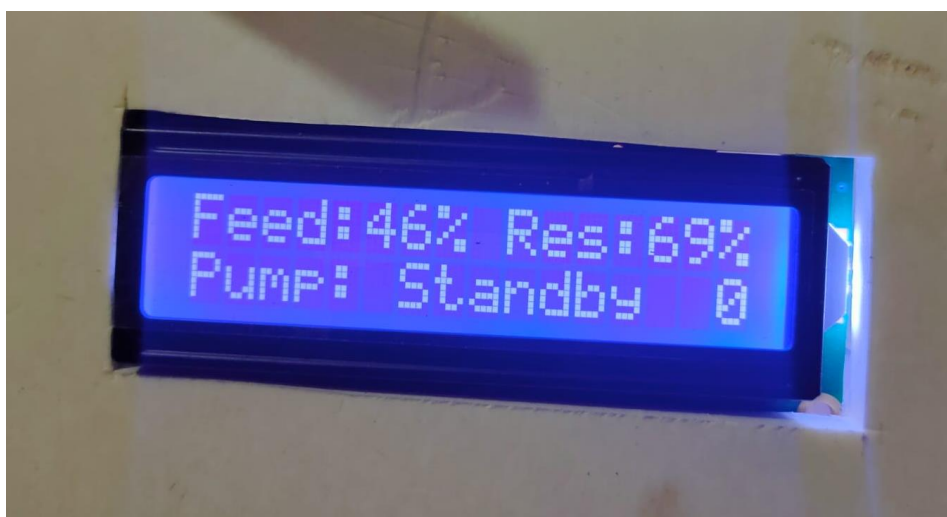
Fig 5.3: System running automatically
