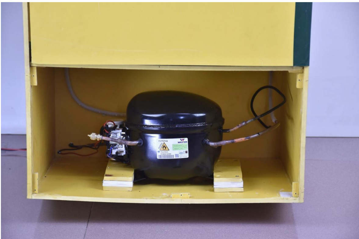
Figureb4.6: Compressor Space
