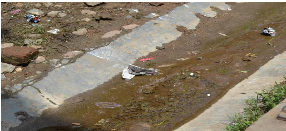
Figure 4- 4.25 Lack of Drainage System
