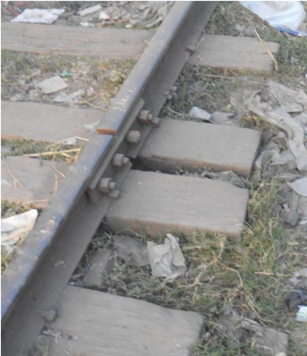
Figure 4- 4.60 Insufficient Stone under Line.
