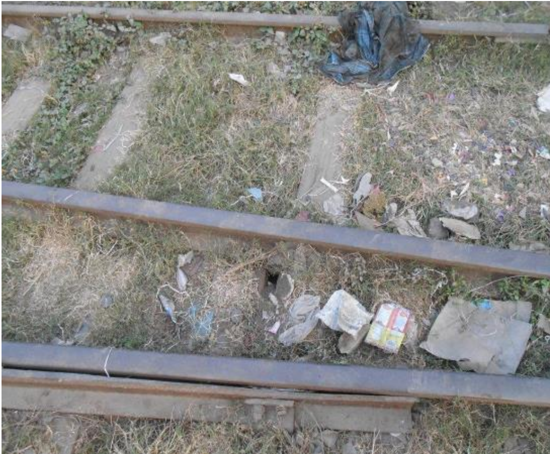
Figure 4- 4.61 Insufficient Stone & weak Wood.
