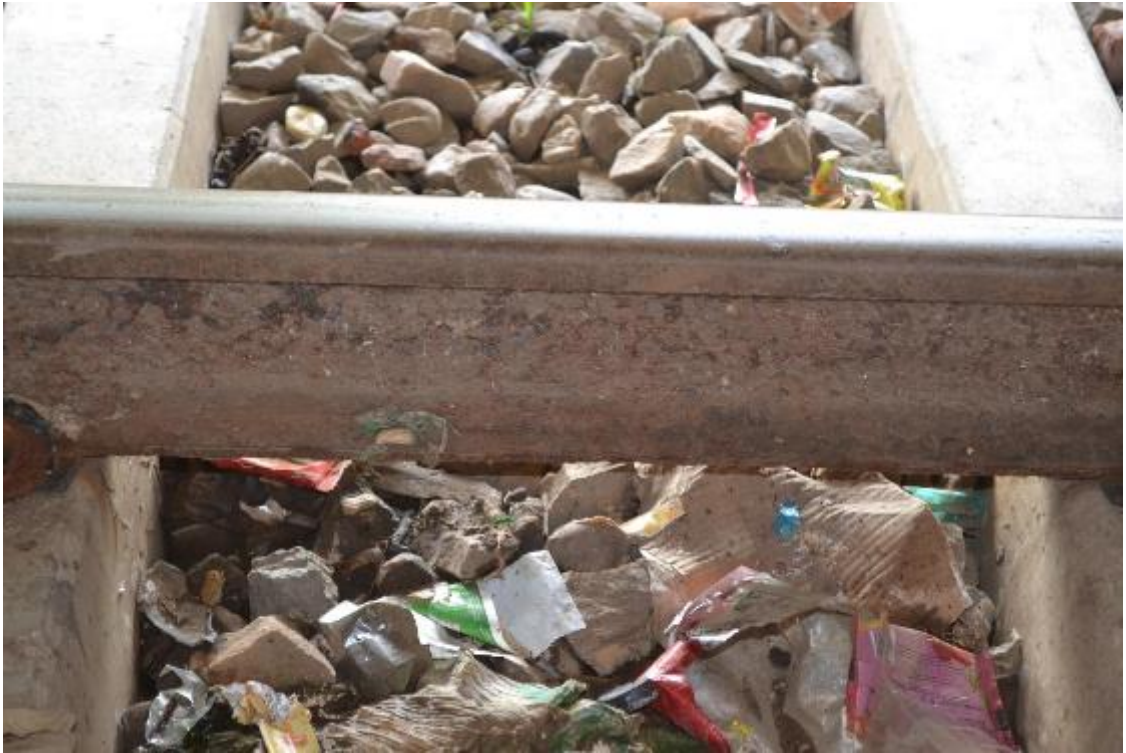
Figure 4- 4.27 No Sufficient Stone under Line
