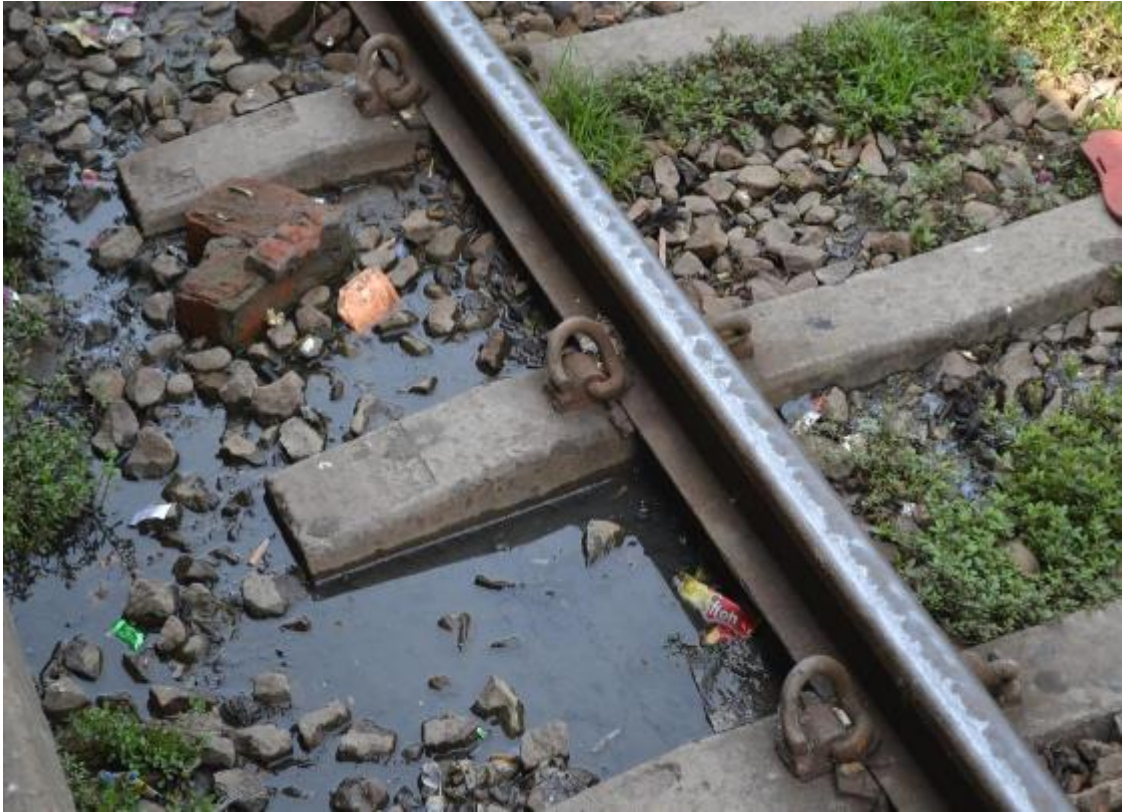
Figure 4- 4.26 Lack of Drainage System
