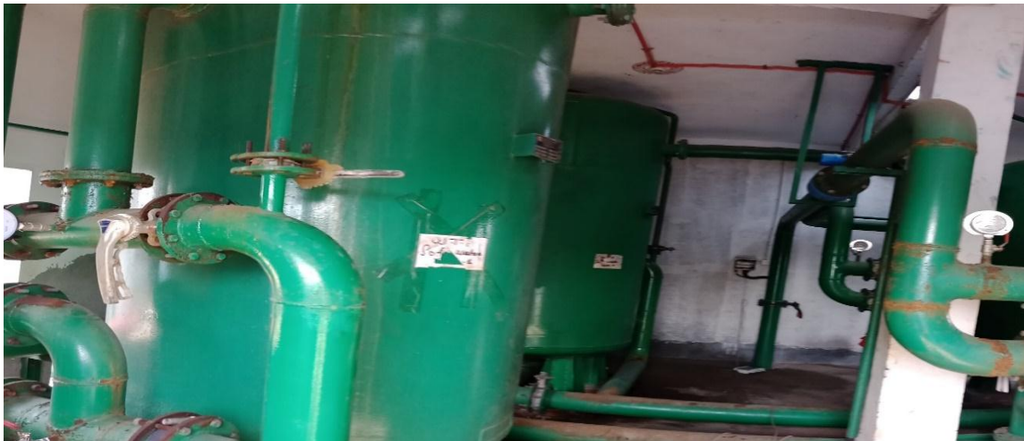
Figure: Water Treatment Plane
