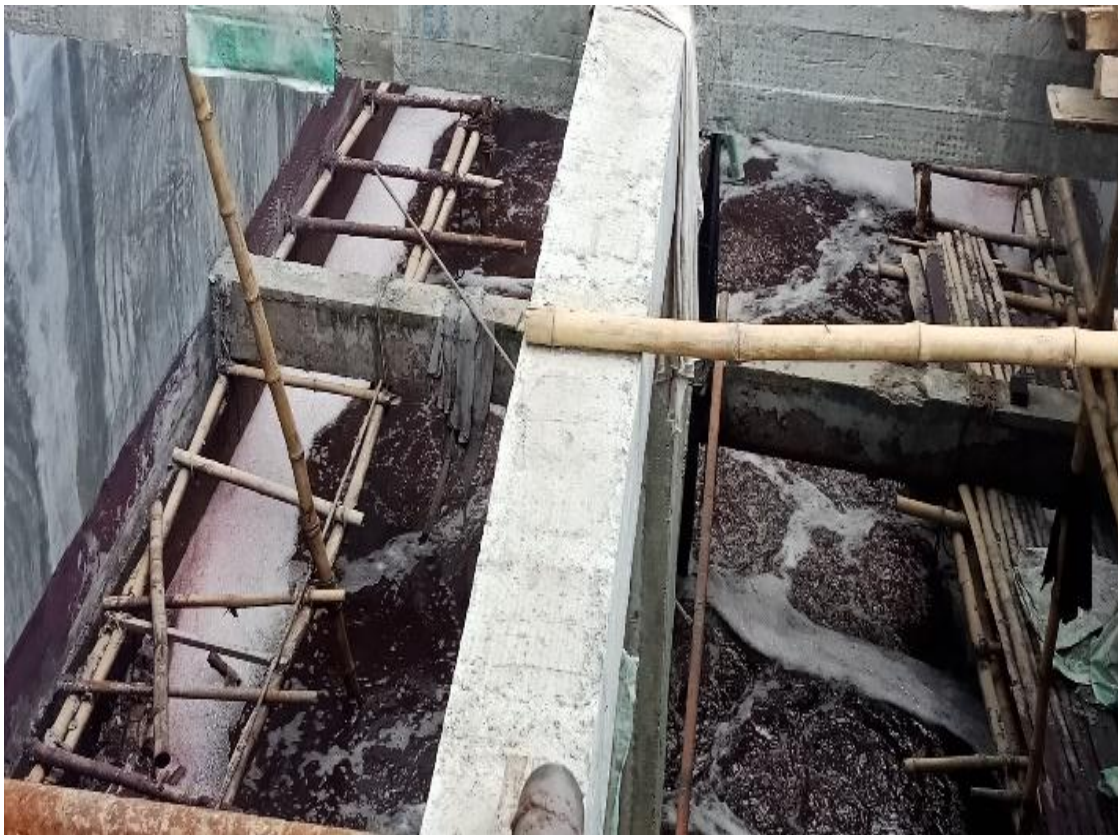
Figure : Screening Unit
