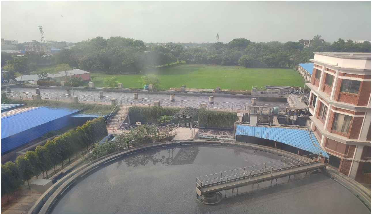
Figure: Water treatment plant
