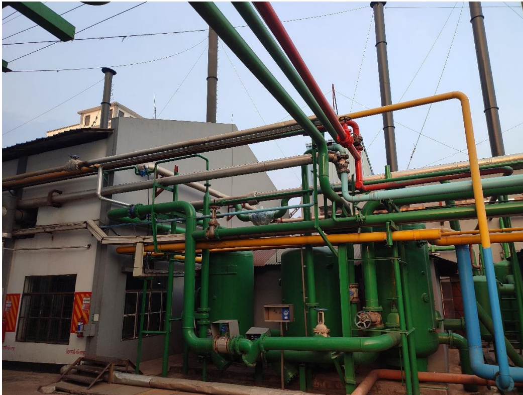
Water Supply Pump
