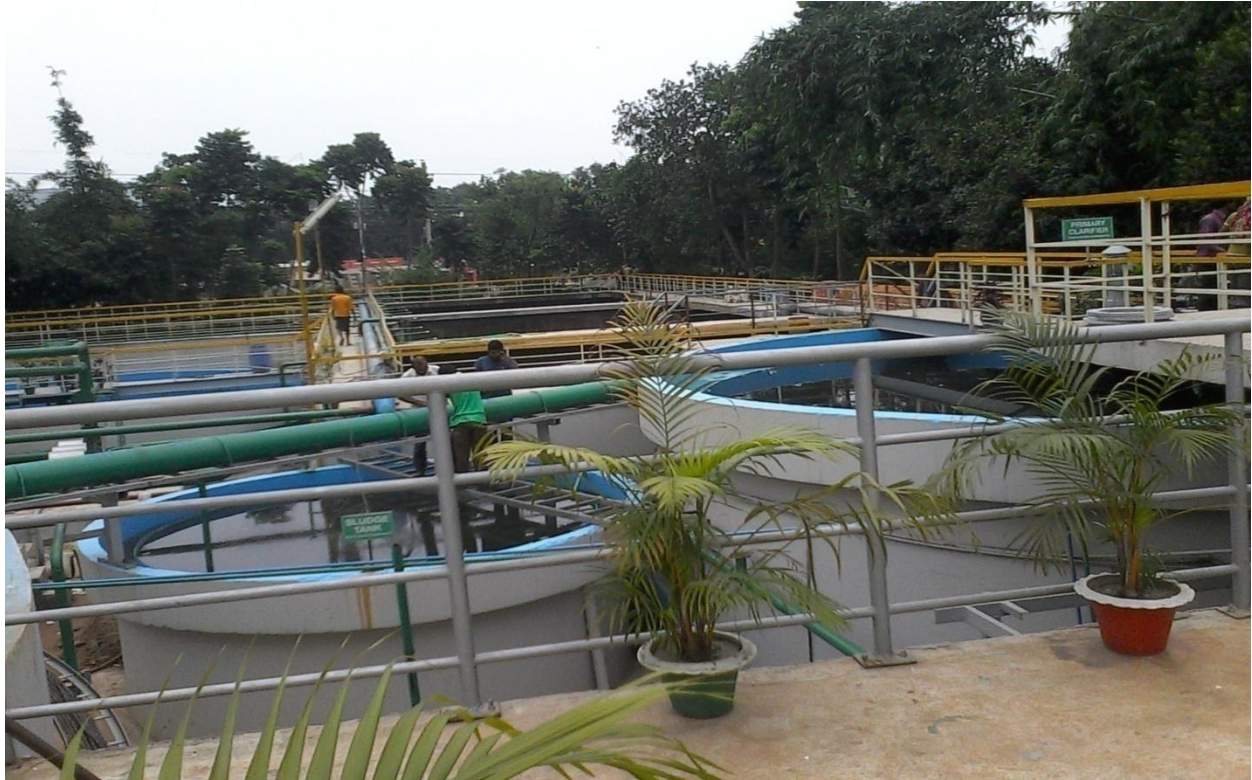
Figure: Effluent Treatment Plant (ETP)
