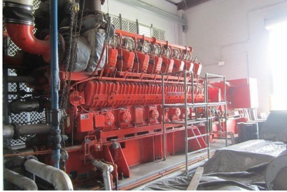
Fig. 8.2 Waukesha Gas Generator
