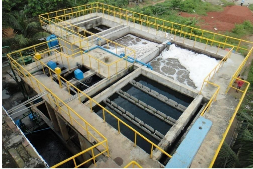
Figure 41: Effluent treatment plant in ADML
