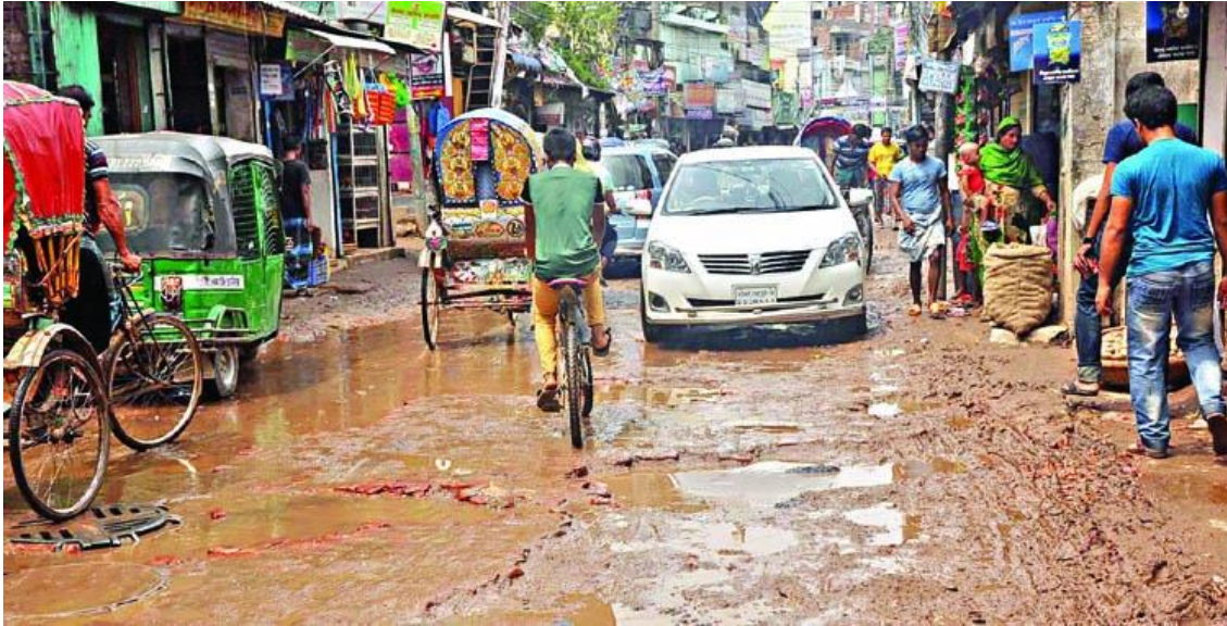
Fig: 4.4 Poor and Dilapidated footpaths and roads
