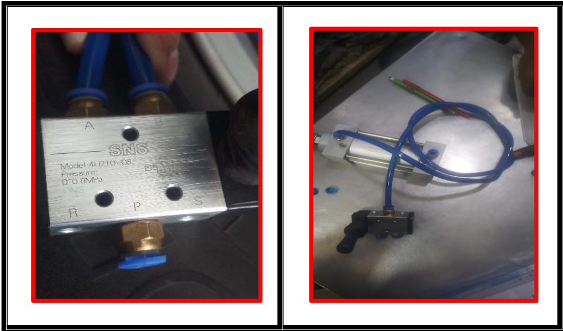
Fig. (c) Solenoid Valve to the Pneumatic Cylinder connectivity (Manual type)
