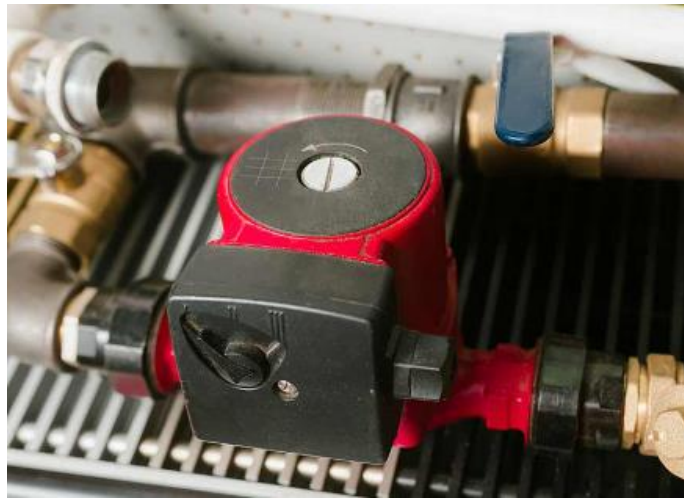
Fig 2.4 Circulating water pump
