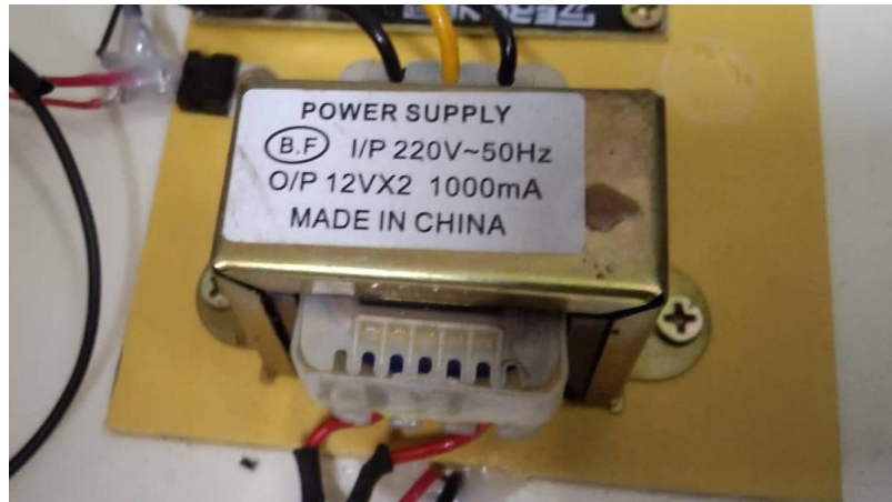
Figure 3.9: Step up Transformer
