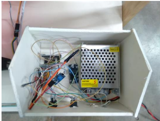
(a) Electrical Components Setup
