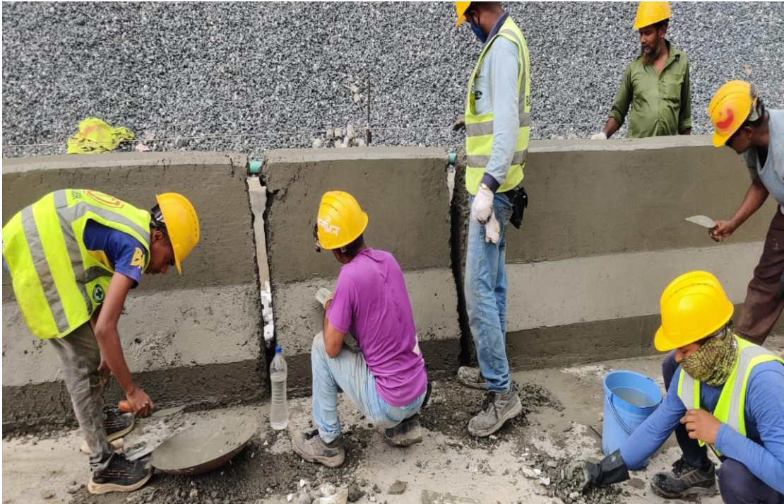
Figure 4-10. Sometimes workers work without proper PPE (FDEE)
