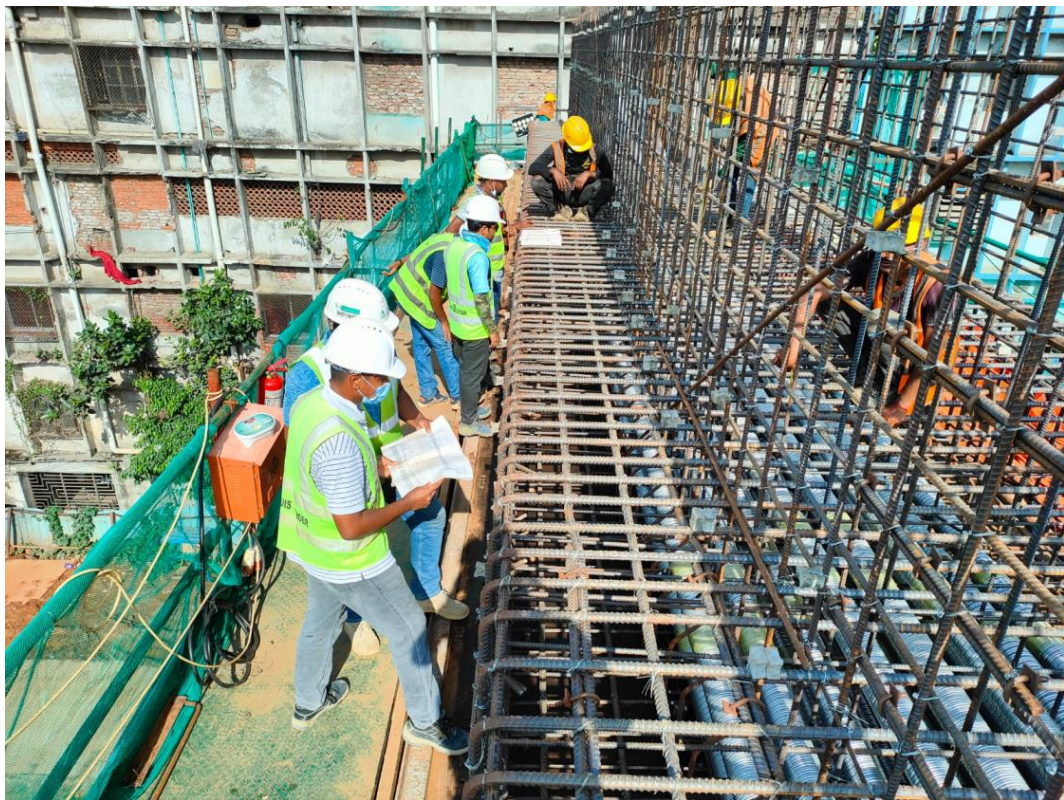
Figure 4-11. Hand rails and nets are used to keep the structure safe from public inconvenience (Dhaka Elevated Expressway)
