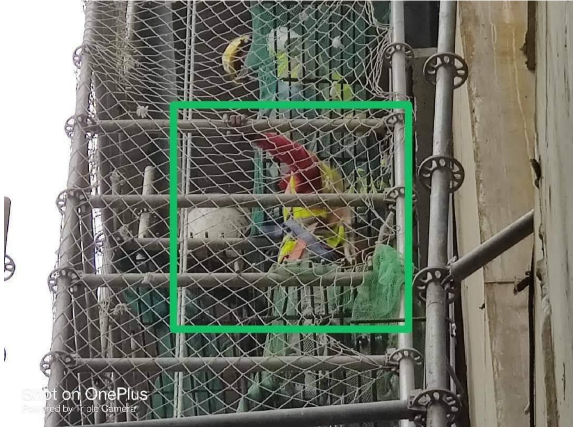
Figure 4-7. Proper PPE and Safety Harness arranged at while working in a height (Line-6)
