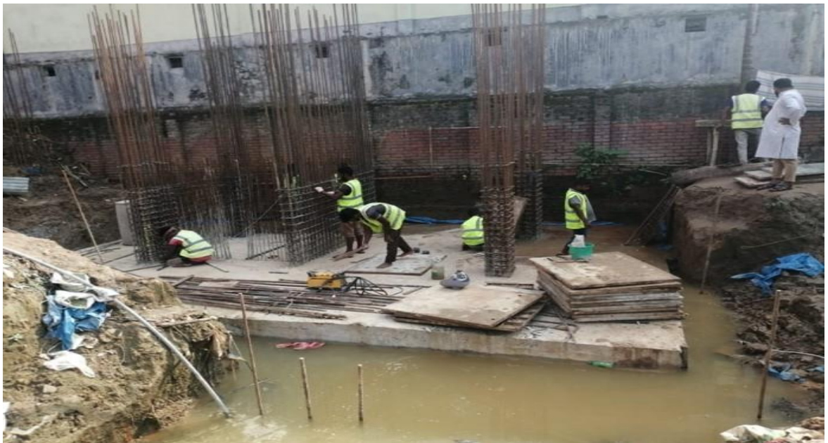
Figure 4-18. Column Casting without safety boots, helmet.
