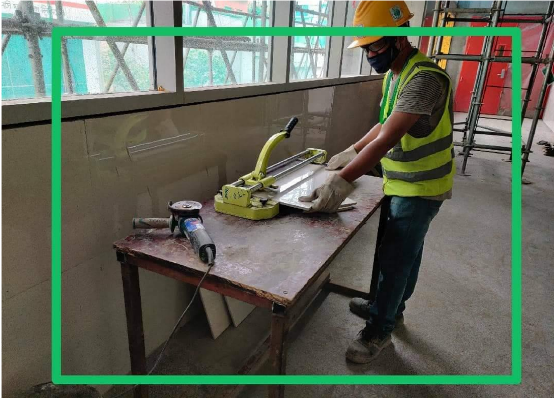
Figure 4-5. Cutting with properly Hand gloves, Goggles and PPE management (Metro Rail, Line-6)
