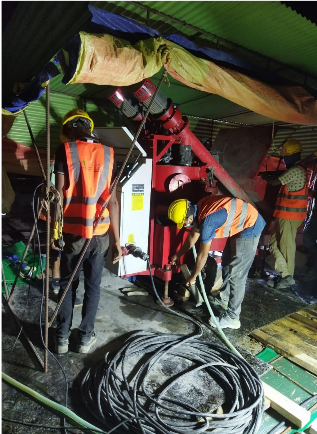
Figure 4-12. Electric machinery and wires should be kept safe and checked (Dhaka Elevated Expressway)
