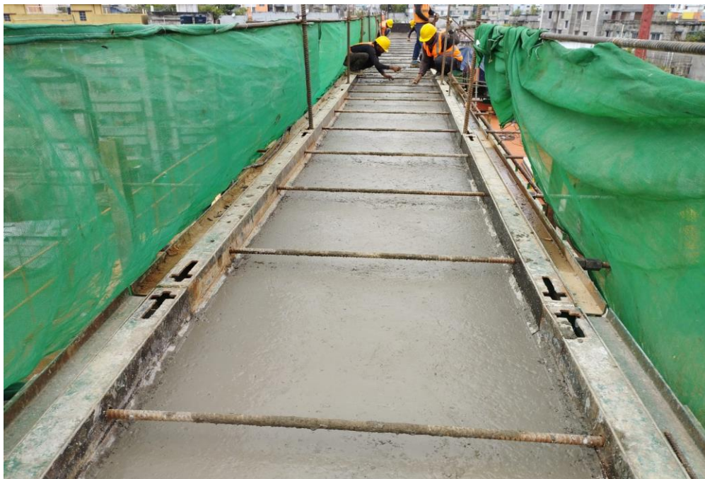
Figure 4-14. Proper fencing is used to avoid any public loss
