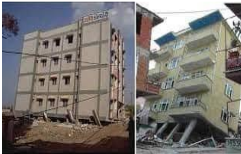
Figure 2.4: Failure of Weak storey building
