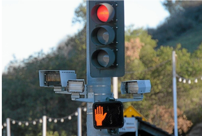
Fig 3.5: Signal mounted video camera for traffic volume count
