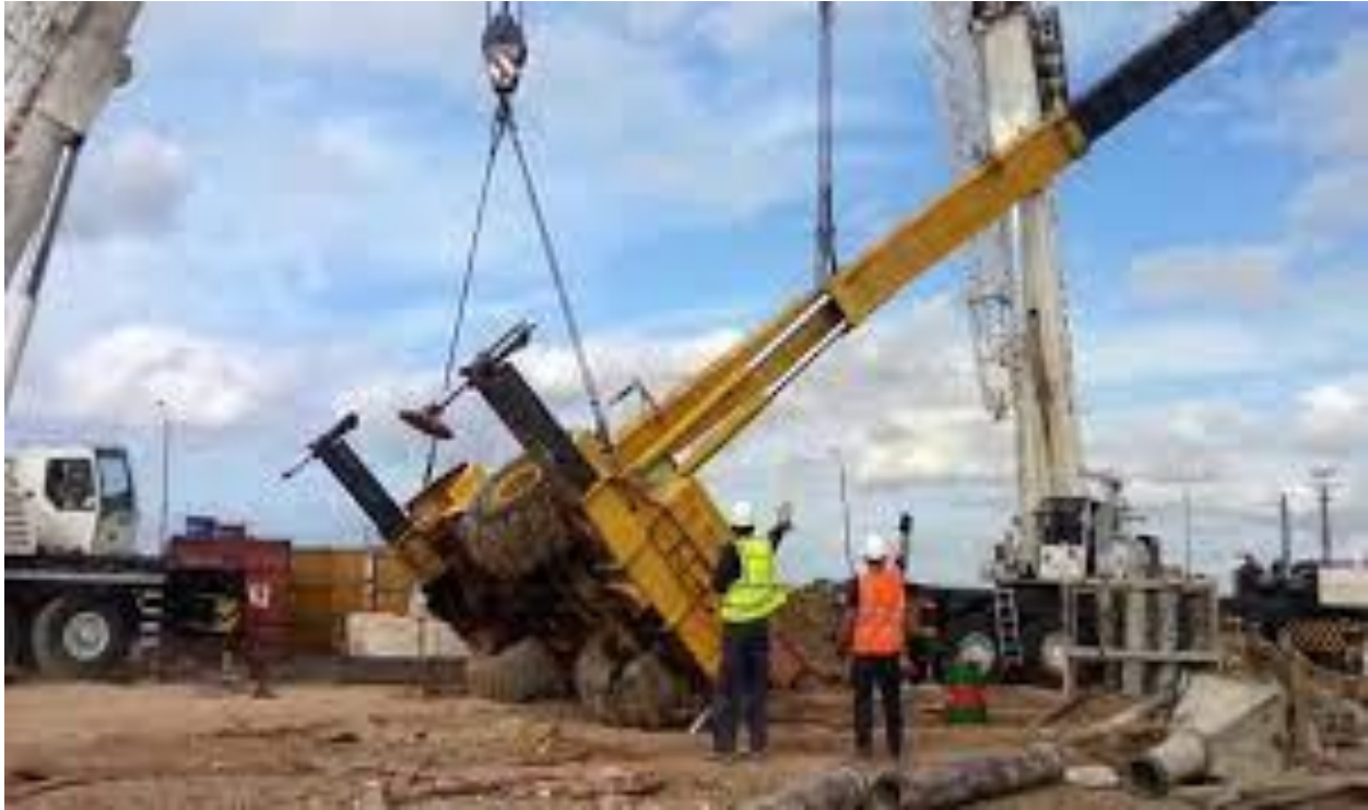
Figure 2.6.7: Vehicle Accident in Construction Sites at Bangladesh.
