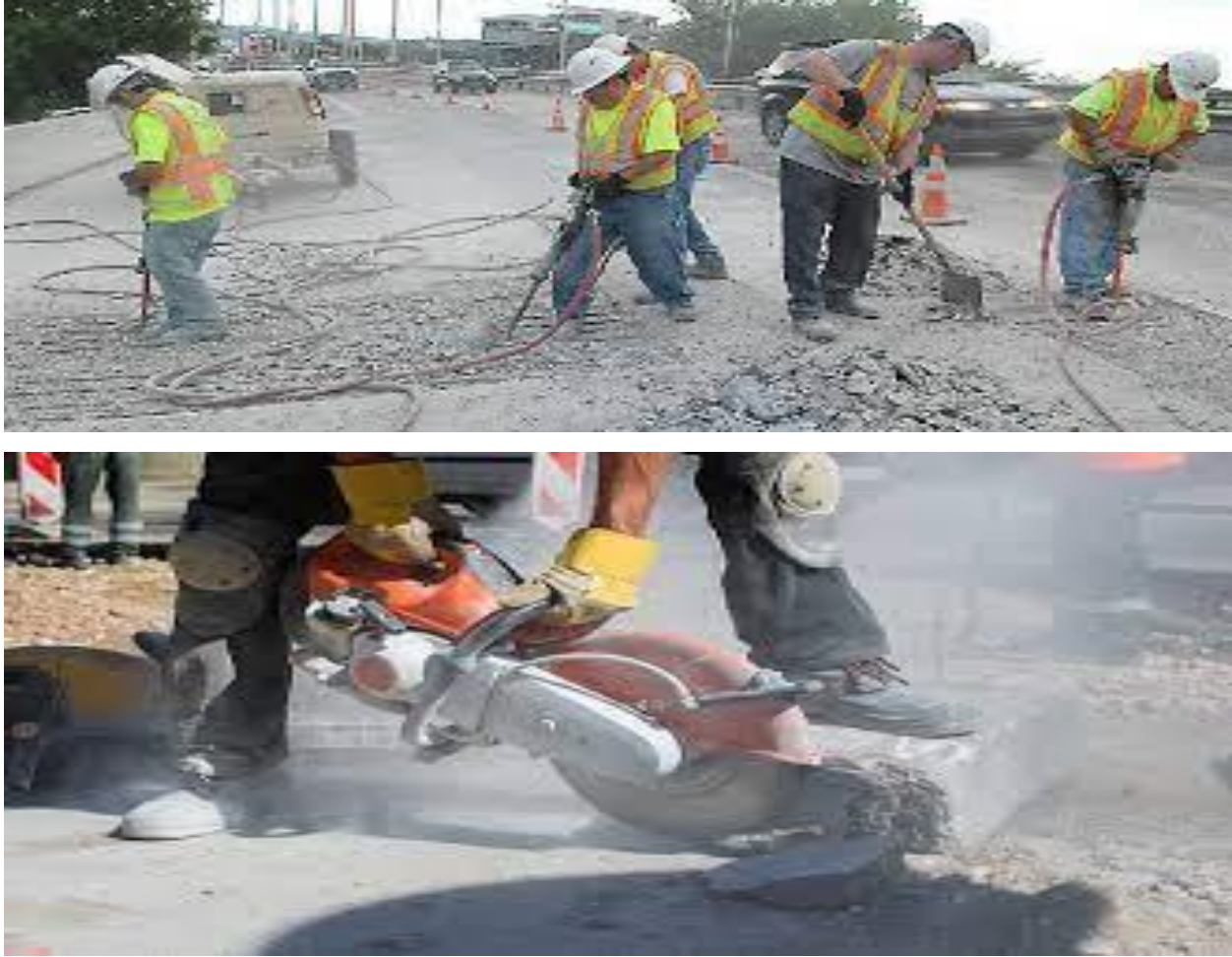
Figure 2.6.6: Excessive Noise and Vibrating Power Tool Hazards in Construction Sites.
