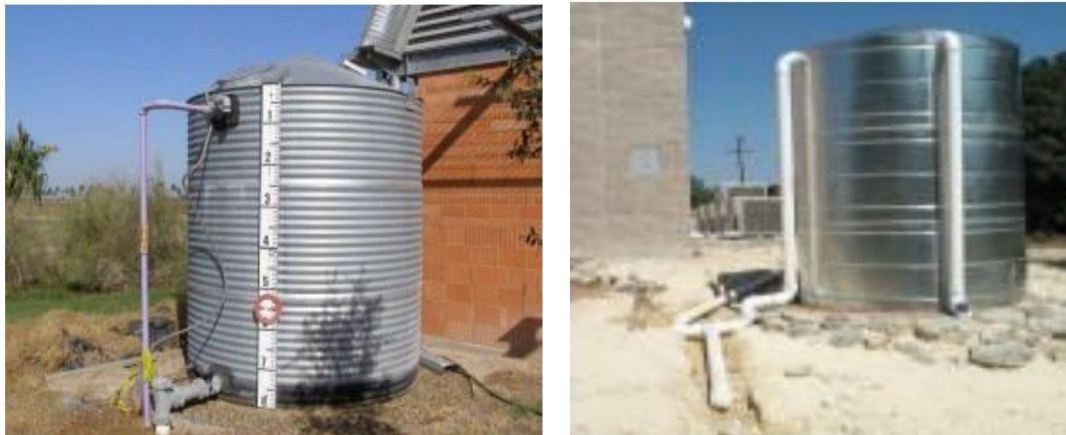
Figure 2-3: Storage container (Steel) [6]
