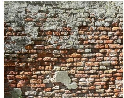
Fig 4.26: Reference Image of Wall after Cleaning Lichen/Algae Growth.
