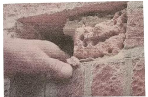
Fig 21: Damage in Brick Wall
