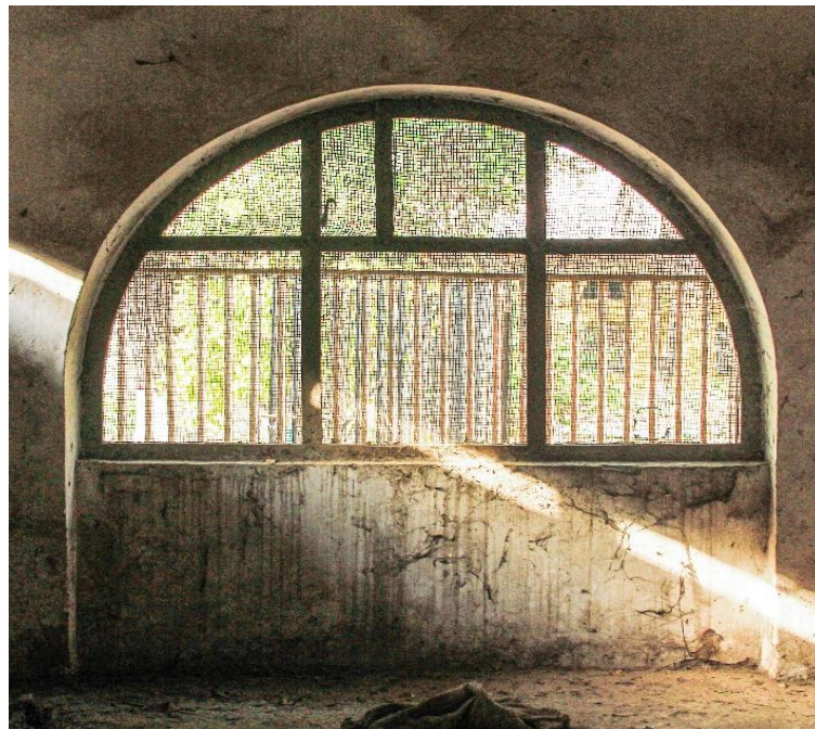
Fig 4.54: Existing Window Condition of CP-05
