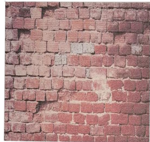
Fig 18: Palling Effects of Bricks
