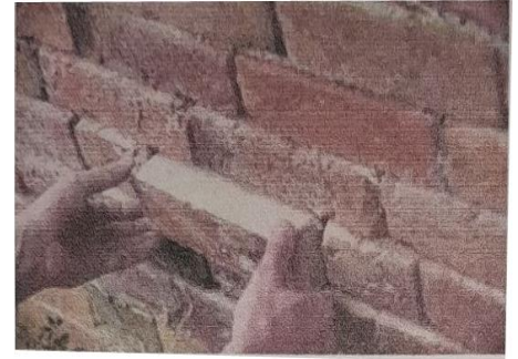
Fig 17: Decayed Bricks in Wall
