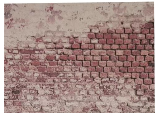
Fig 19: Cracks in Brick Wall
