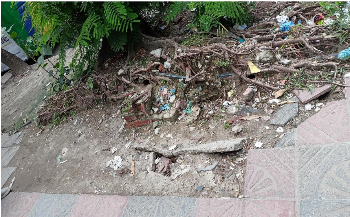
(c) Broken segment of footpath
