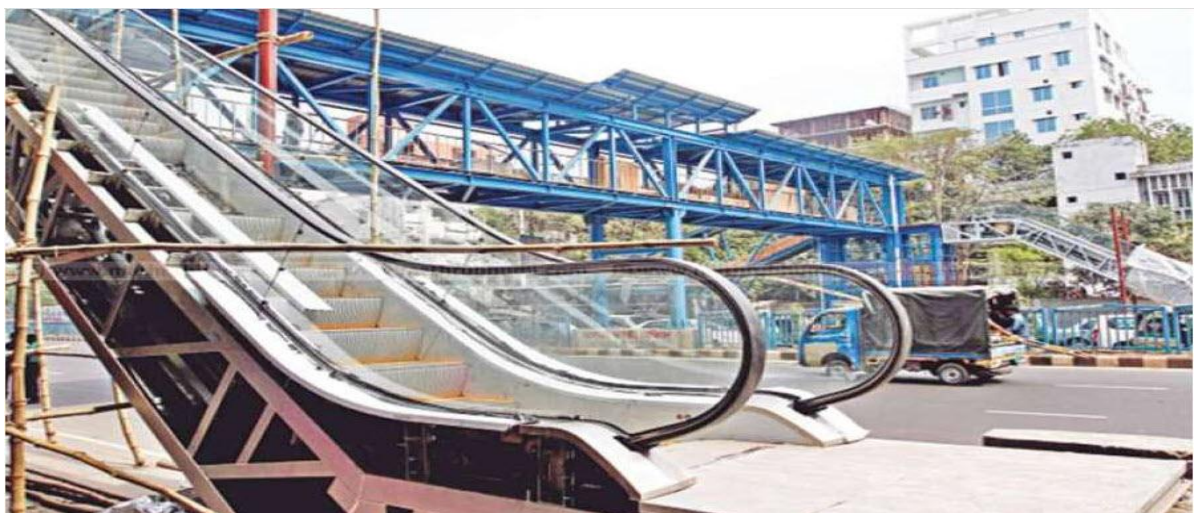
Figure 15: Banani Foot over bridge escalator one sided setup (5)
