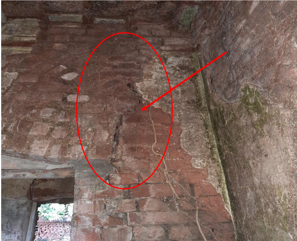
Figure.4.6. Vertical crack of wall.
