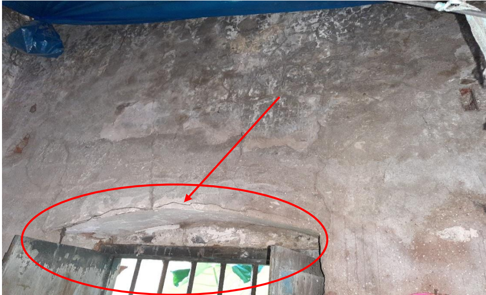
Figure.4.4. lintel joint crack
