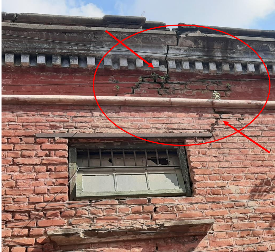
Figure.4.14. Crack on due to settlement failure.
