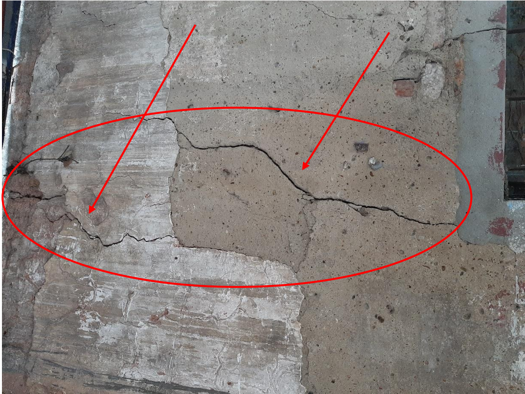
Figure.4.16. Crack on due to the deformation of support.
