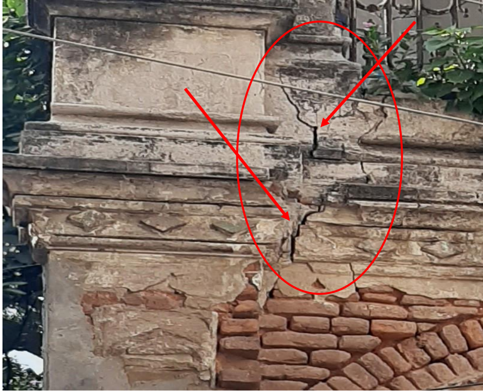
Figure.4.20. Crack on due to the Joint failure/share failure.
