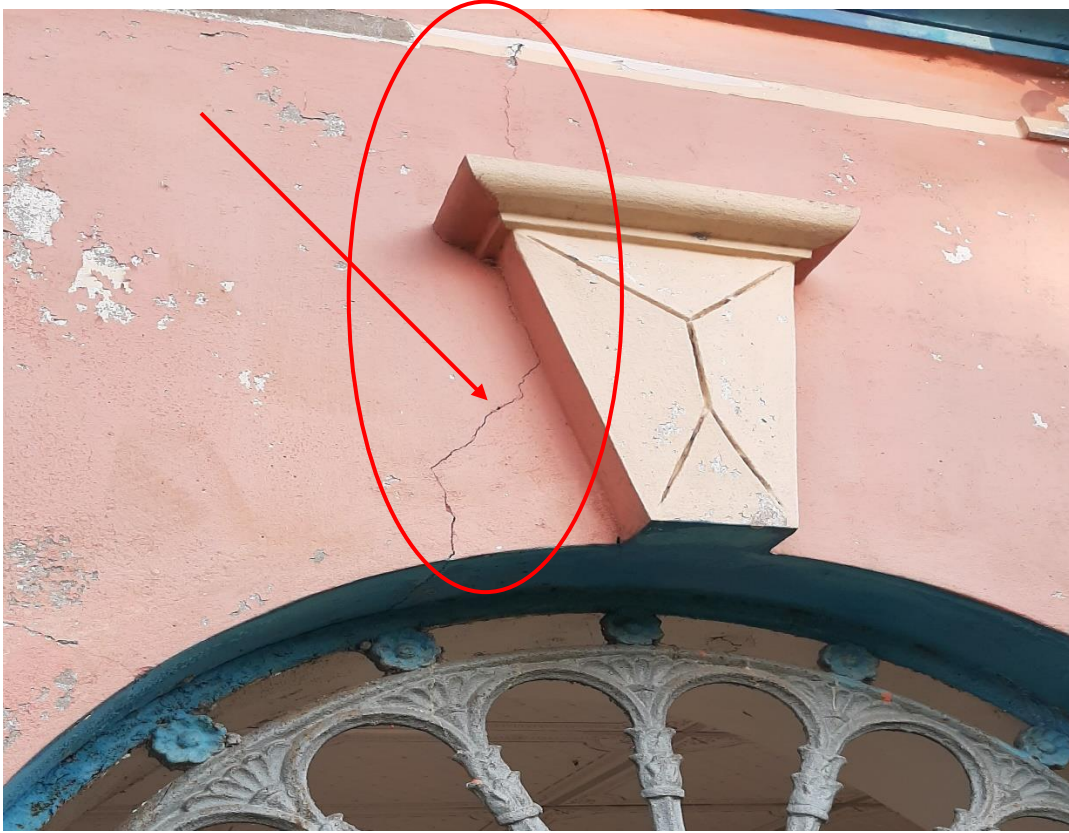
Figure.4.10. crack on due to settlement failure.
