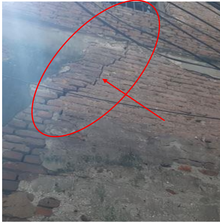
Figure.4.18. Crack on due to the masonry settlement.
