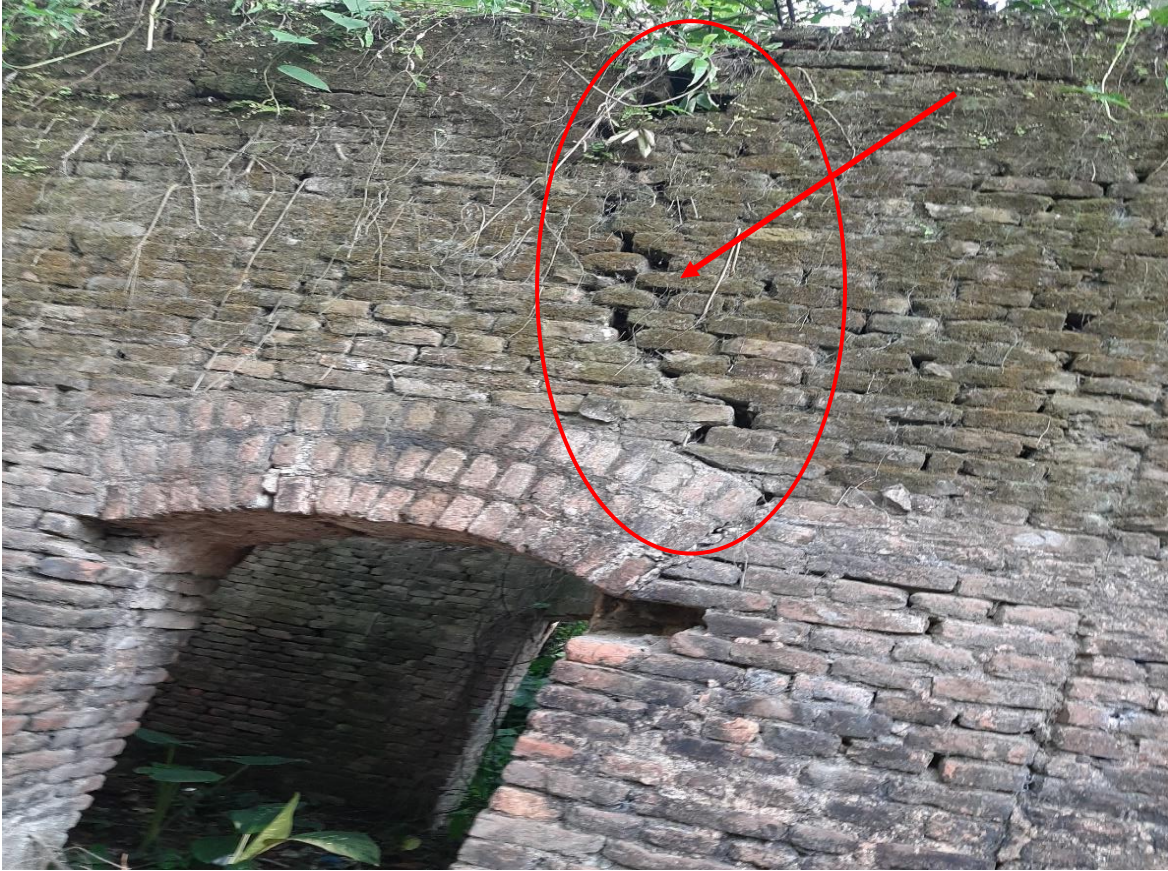
Figure.4.8. crack on due to differential settlement of structure.
