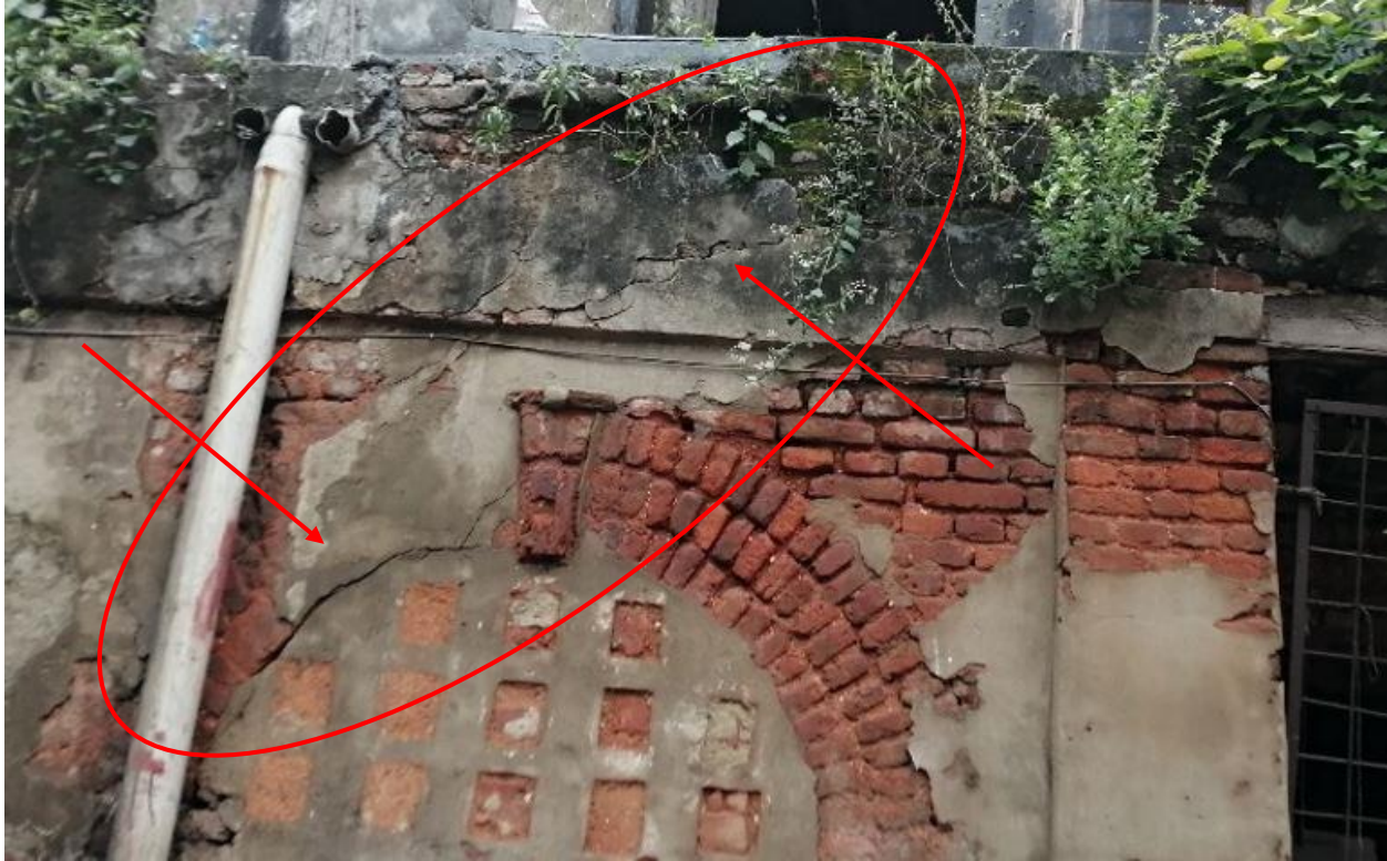
Figure.4.12. Crack on due to ageing impact/ settlement failure.
