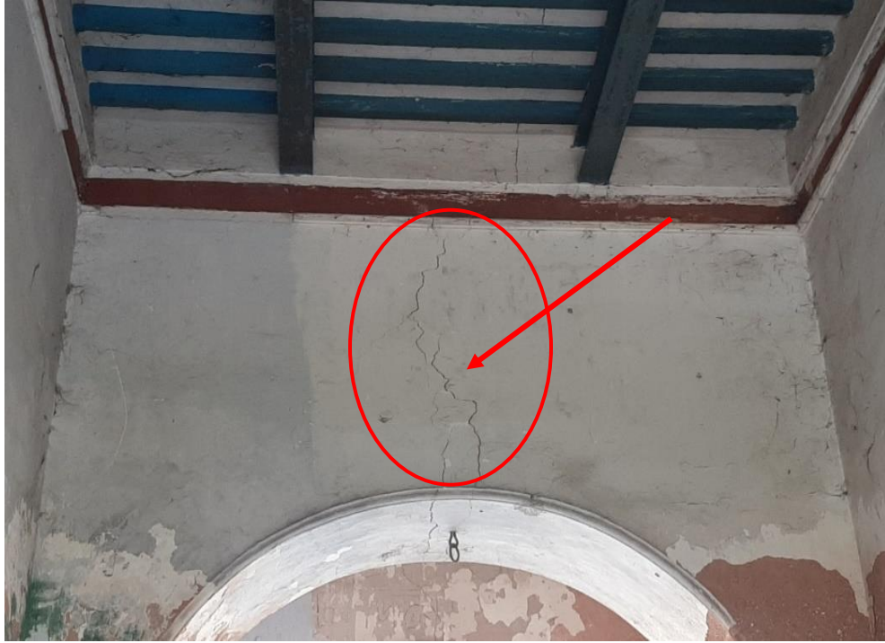
Figure. 4.2. Picture of arch crack
