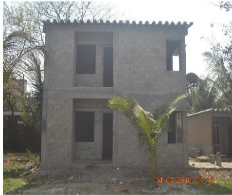
Figure 1.3: Model House-II using Compressed Stabilized Earth Block and Thermal Block at HBRI campus
