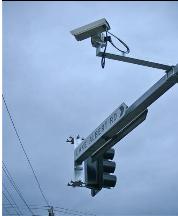
Fig 2.5: Signal Mounted Video Camera for Traffic Volume Count
